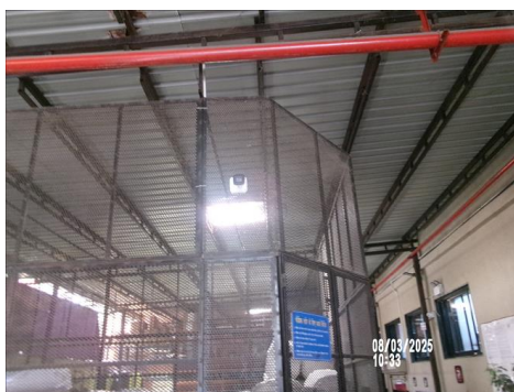
CCTV at loading area
