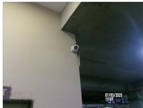
CCTV at parking
