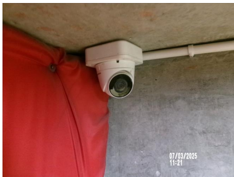
CCTV at packing
