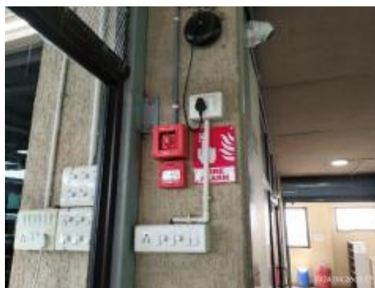
Manual Call point in first floor.jpg
