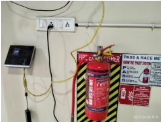
Fire Extinguishers with working instructions.jpg
