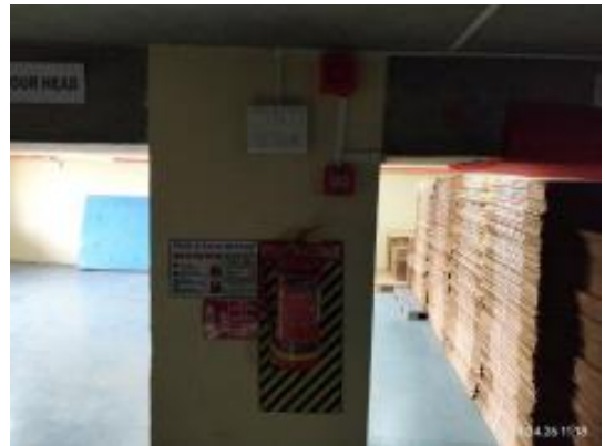
Fire alarm call point with alarm.jpg
