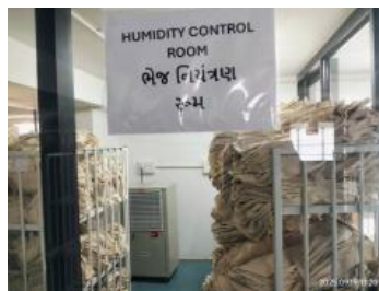
Humidity control Room.jpg
